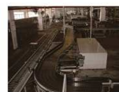
Steel slat C/V transferring line
