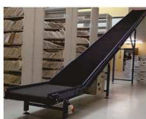
Inclined conveyor in storehouse
