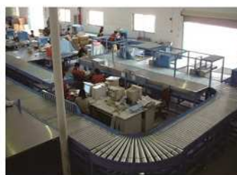
33. Package distribution line with roller conveyors
