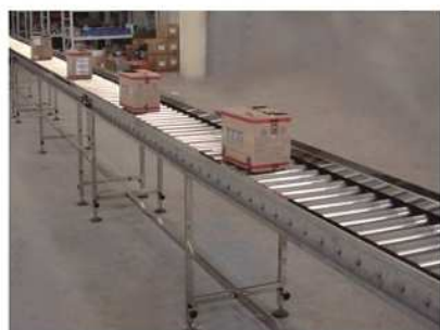
Conveyor line in full stainless steel structure
