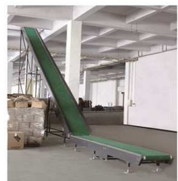
Inclined belt conveyor between floors
