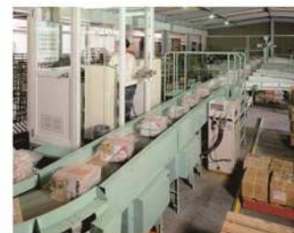
32. Package distribution line on belt conveyors
